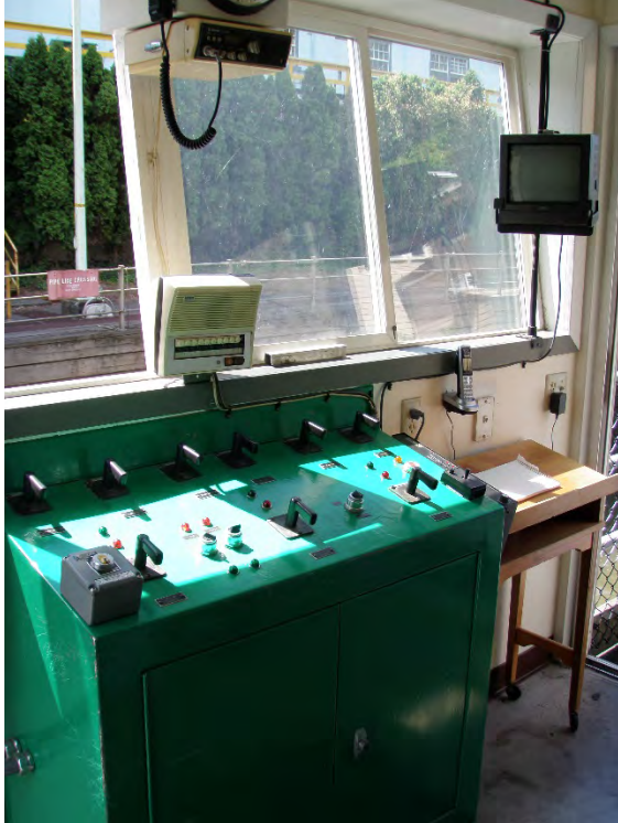
Figure 10: View of Controls and Communication Mechanisms Within the Lock Control Stand at Gate 4
